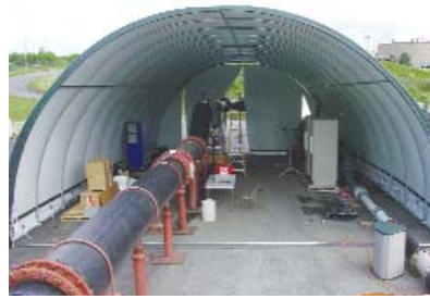
While the existing validation facility was originally limited to testing 8- and 24-mgd UV units, it will test 60-mgd units once expanded.
