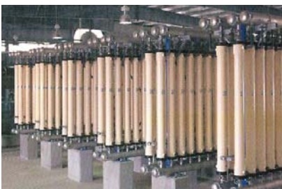
One of the keys to success is understanding system differences. Shown above are three of the many available systems: 1) US Filter CMF-S system (at 33-mgd Coliban WTP, Australia); 2) Zenon ZW500 system (at iron removal plant, Seekonk, MA); and 3) Pall Aria MF system (at 5.2-mgd WTP, Ingleside, TX).
