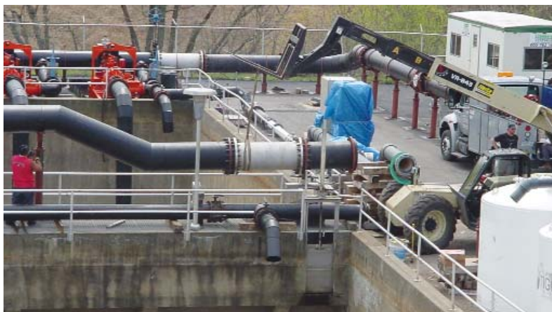
Validation for NYC's 2,020-mgd UV facility will be conducted at this testing facility in Johnstown, NY, which is being constructed/expanded to accommodate this effort.
