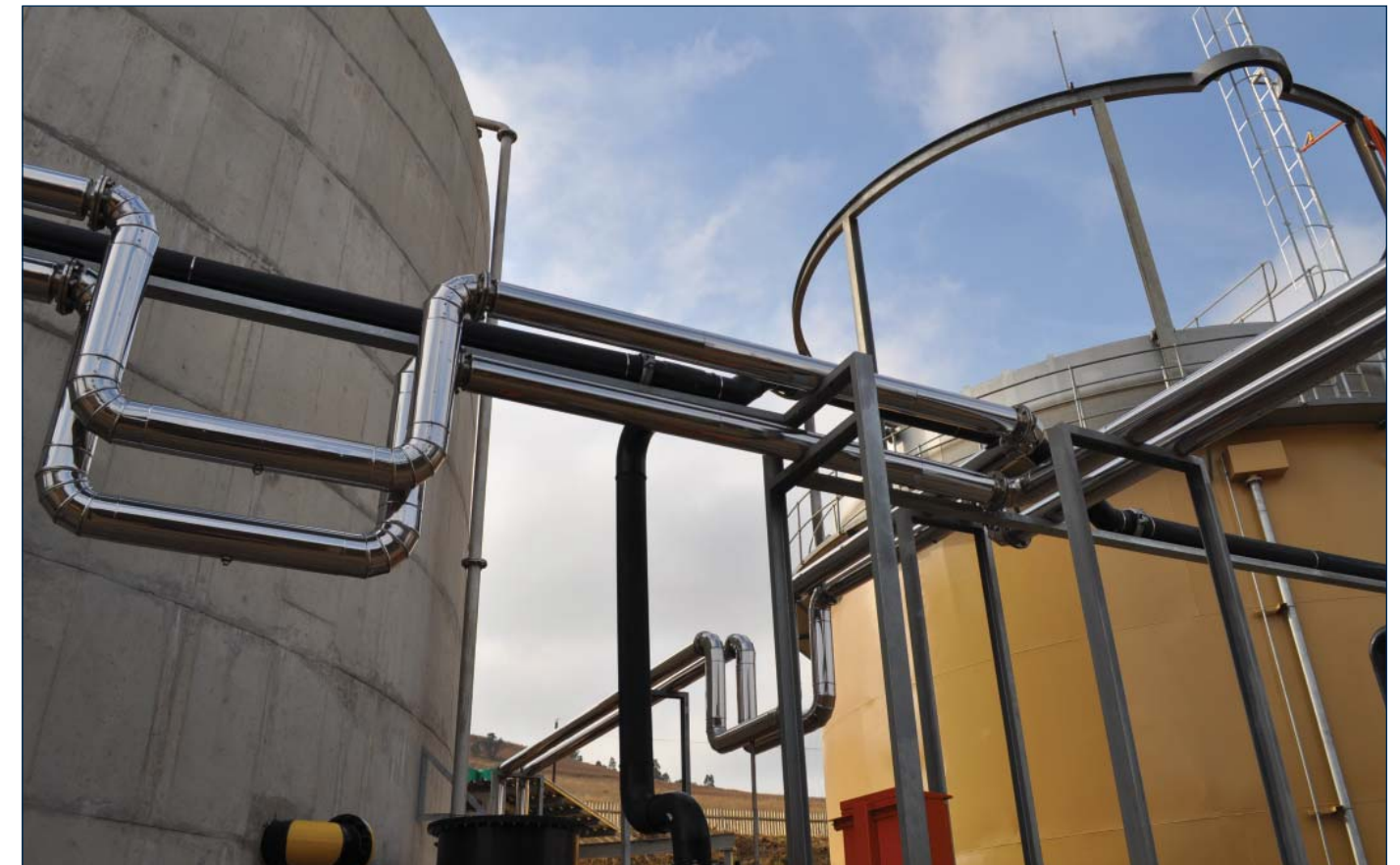
With energy costs on the rise, the Driefontein WWTP is among five facilities adding high-performance mesophilic anaerobic digestion to their process, increasing biogas production for use in generating power and lowering energy costs.
