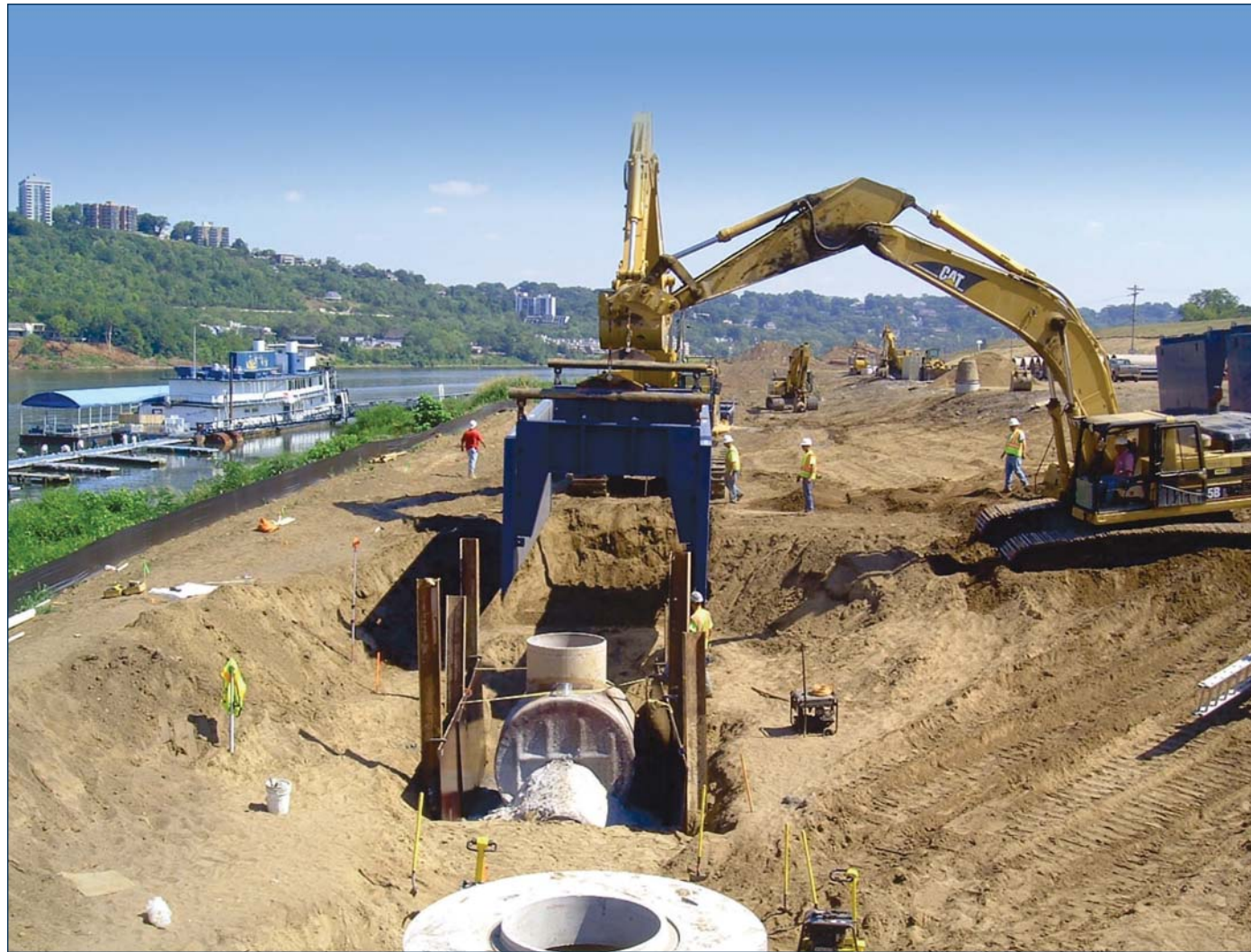
Construction of the replacement in-line storage interceptor is nearing completion. This project is projected to result in a reduction of 56 million gallons of CSO annually, and will significantly reduce solids and floatables discharges to the Ohio River during very large storms.
