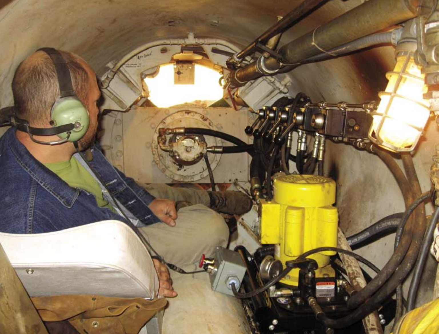
An operator at the leading edge of the casing. The cutting head is visible in the background.
